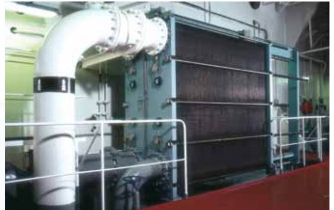
Main engine lube oil cooler
