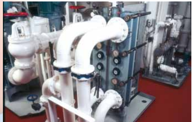
Stern tube lube oil cooler
