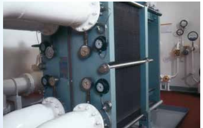
Jacket water cooler
