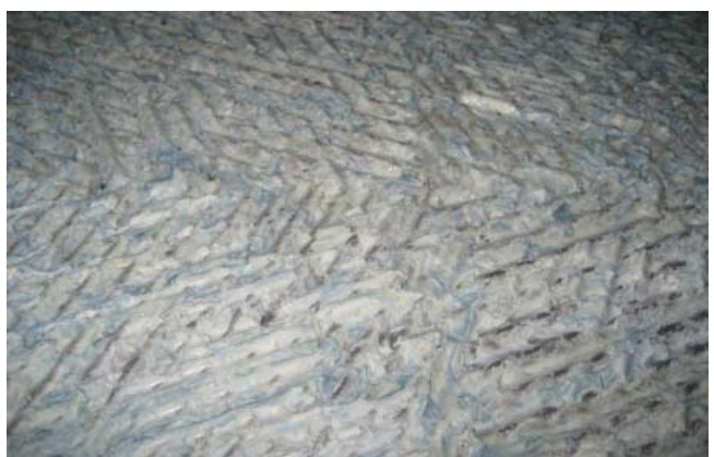
Limescale can block your heat exchanger.
