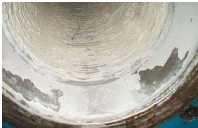
Crystallisation of fluids when they get in contact with oxygen can deform and damage the plates.
